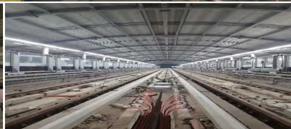
Platform Level Lighting at Doordarshan Kendra
