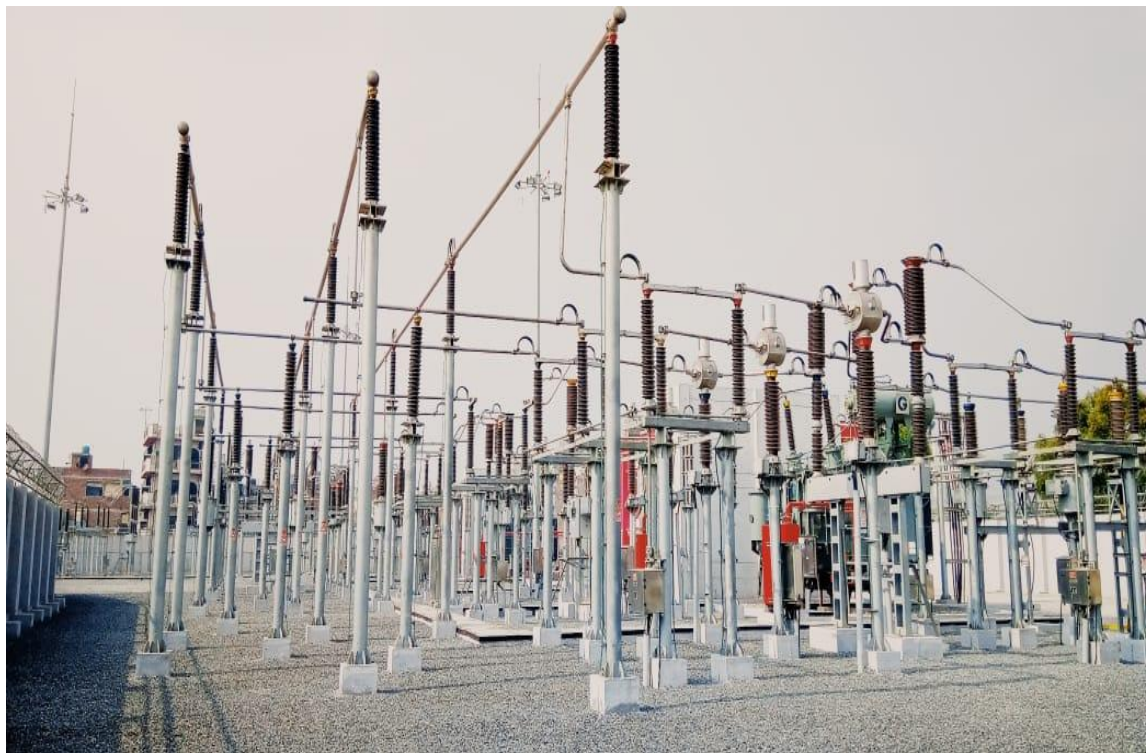
Figure 10.2: Photograph of a Typical Air Insulated Receiving Substation (AIS)
