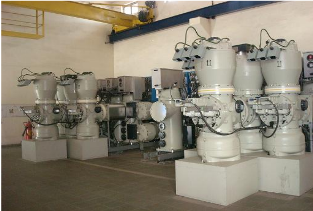
Figure 10.3: Photograph of a Typical High Voltage Gas Insulated Switchgear
