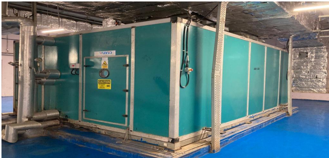
Air Handling Unit
