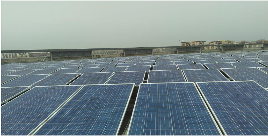
Figure 10.13: Solar PV Power panel
