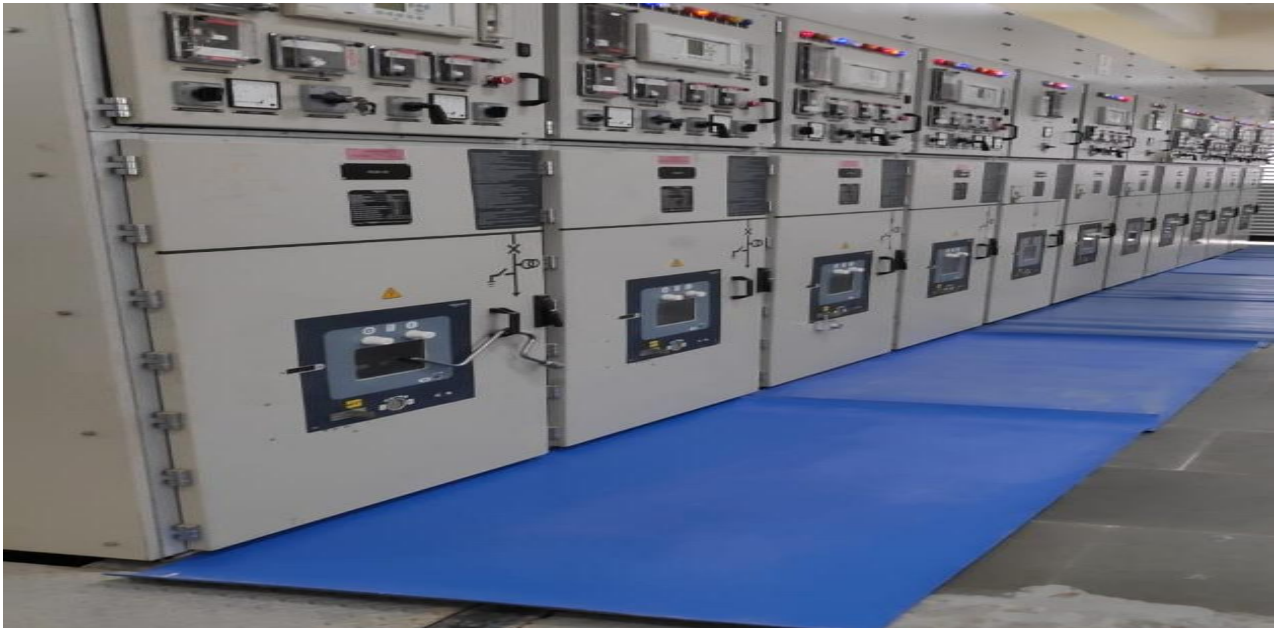
Figure 10.11: Typical Indoor Auxiliary Sub-station
