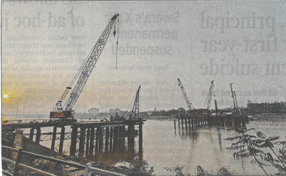
Construction of the bridge for the metro line between Adajan and Athwagate is in full swing
