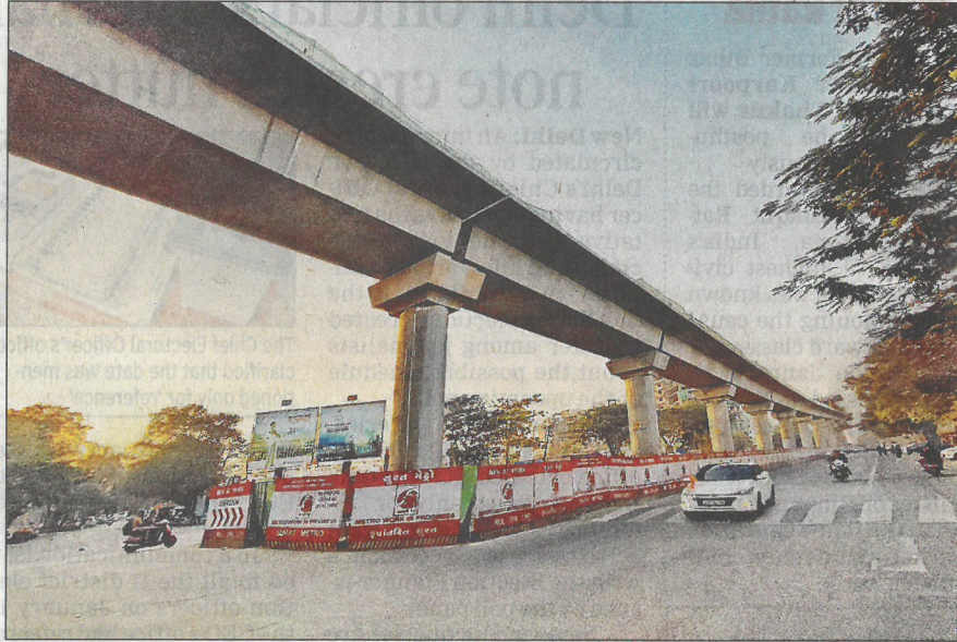
Work for metro rail project in full swing on L P Savani road in Pal area of Surat
