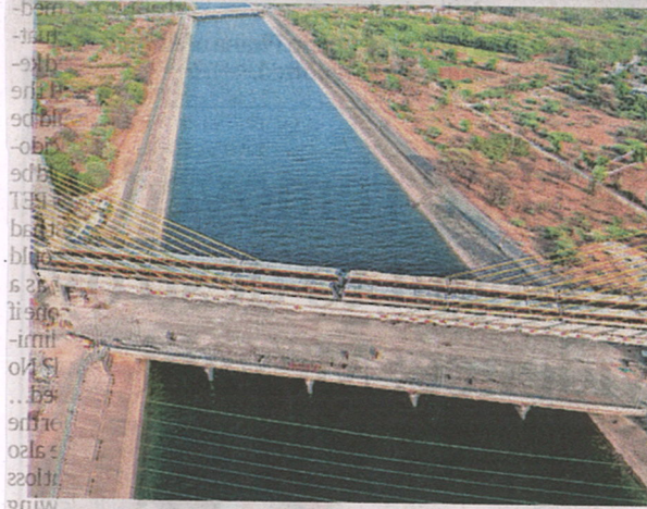
Metros run on the cable-stayed bridge over Narmada canal as part of the load test. Express
